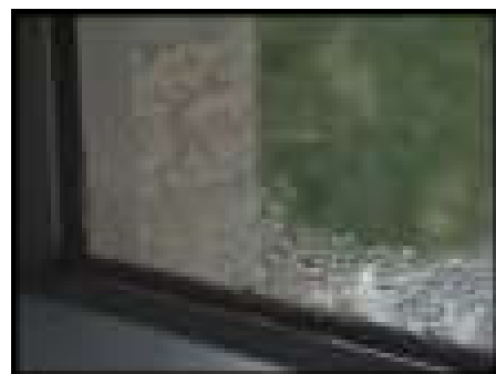
Condensation on windows
