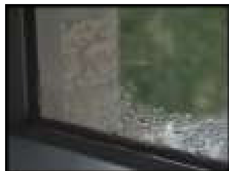
Condensation on windows
